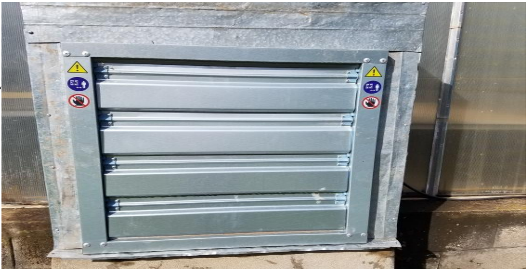
Fig.42. New greenhouse fans purchased and the motors of old fans rewired
